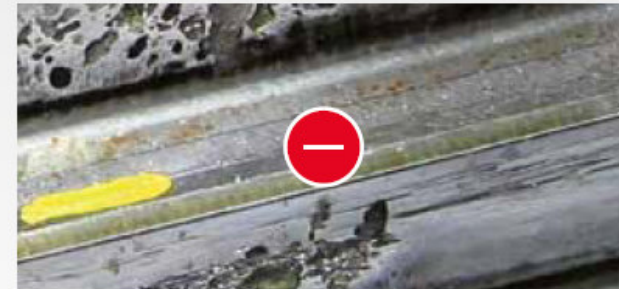
Sharp edges and pittings: the applied gearbox oil was not up to the typically prevailing loads.
